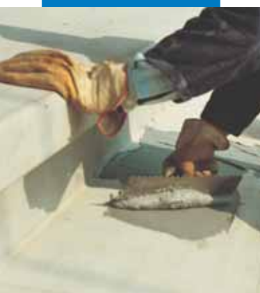
Application of Adesilex PG1 with a notched trowel for structural bonding of pre-fabricated steps
