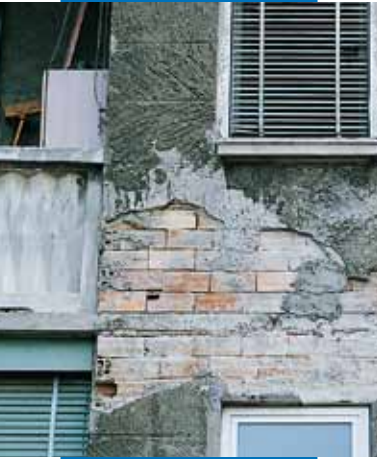
Degraded building façade in need of repair
